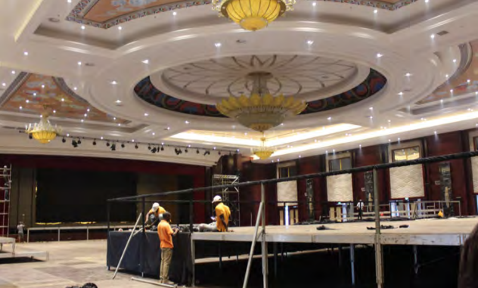
Renovations at the Gloria Hotel in Maputo, meeting place of the Mozambican elite and international visitors (photo Estacio Valoi)
